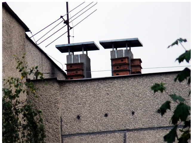
Fig. 10. Nesting boxes for swifts hung too low above the roof. There is no chance on their inhabiting by swifts
