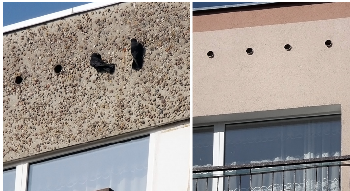
Fig. 1. Inlet tubes installed in the roof structure inhabited by Jackdaws should provide an easy access to the birds' habitat after the renovation - in this building (left – before renovation; right – after renovation) the Jackdaws lost their habitat due to the installation of smaller diameter tubes than the recommended 93 mm
