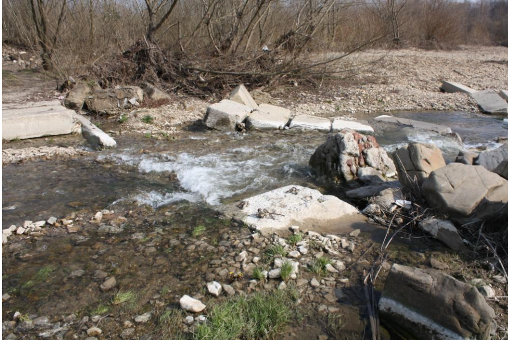
Figure 4. Destroyed gabions because of intensive vertical deformation of the riverbed (March 2016)
